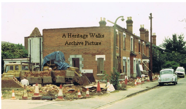
This one, obviously taken with the 'SLR', shows the demolition of the houses of Butts Road, off Goldsworth Road in August 1981.
