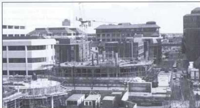
The construction of the new Library (left), with Barclay's Bank (centre) and the hoarding around Christ Church (right).
