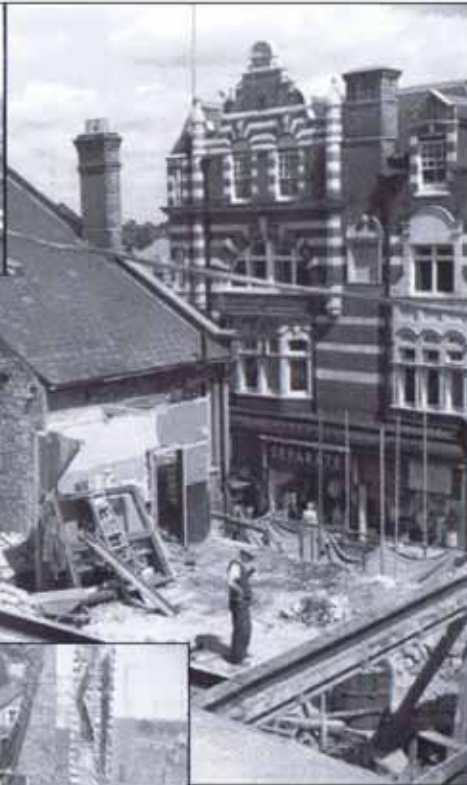
The building of the new Woolworth's store (now part of Weatherspoon's) in 1958.
